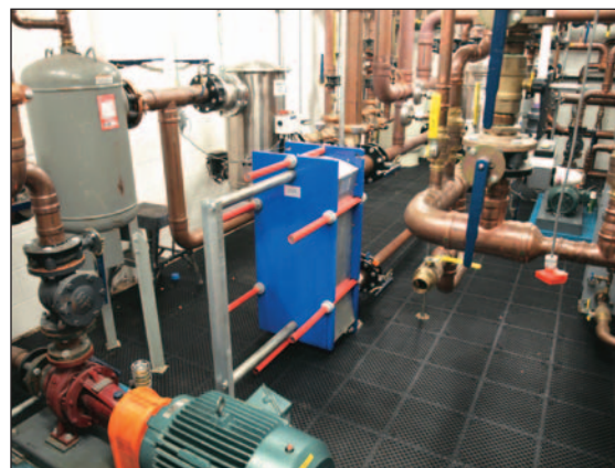
This blue suitcase-sized heat exchanger replaced a 340 ton chiller!
